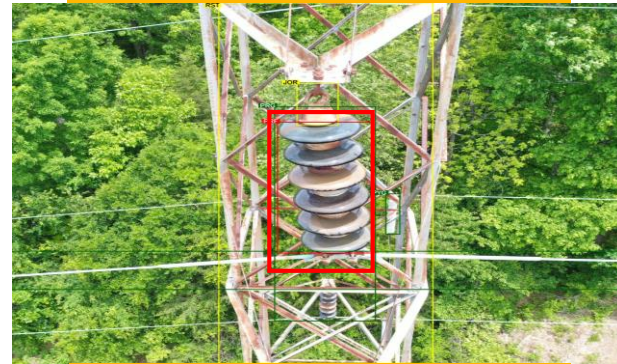
Insulator Flashing, Rusted C-Hook, Structure Rusting
