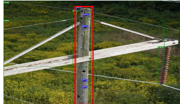
Pole Cavities and Cracks
